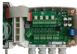
The relay module is properly installed and functional.
